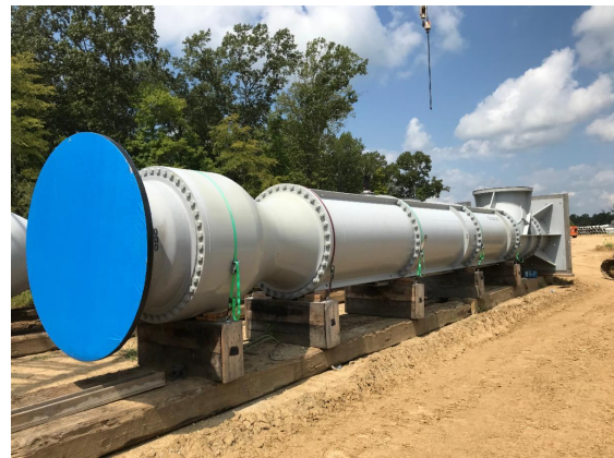
One of Four Booster Pumps
